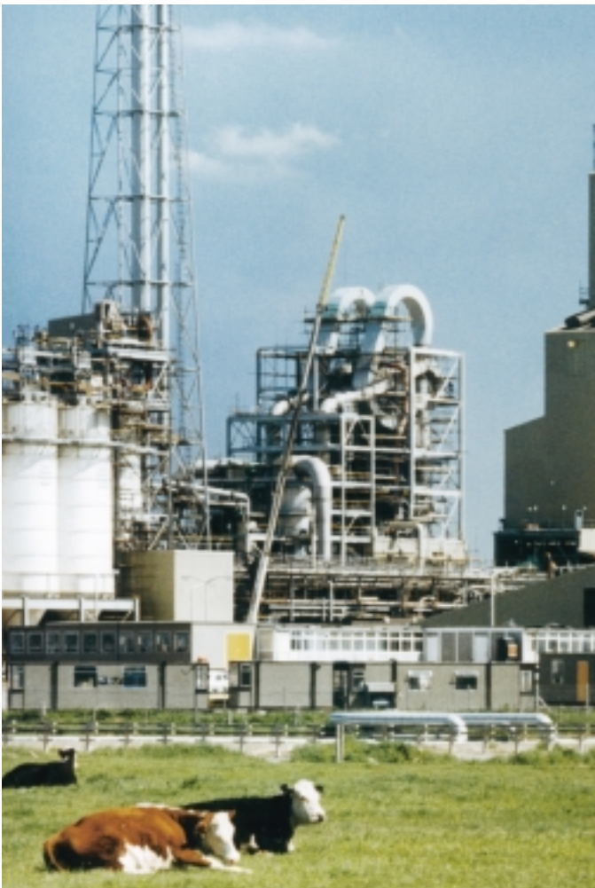
Two flash dryers rated for 15 t/h evaporation
