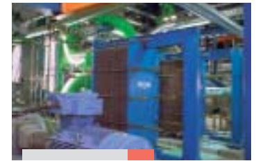
Vasa Power station, Cottbus
